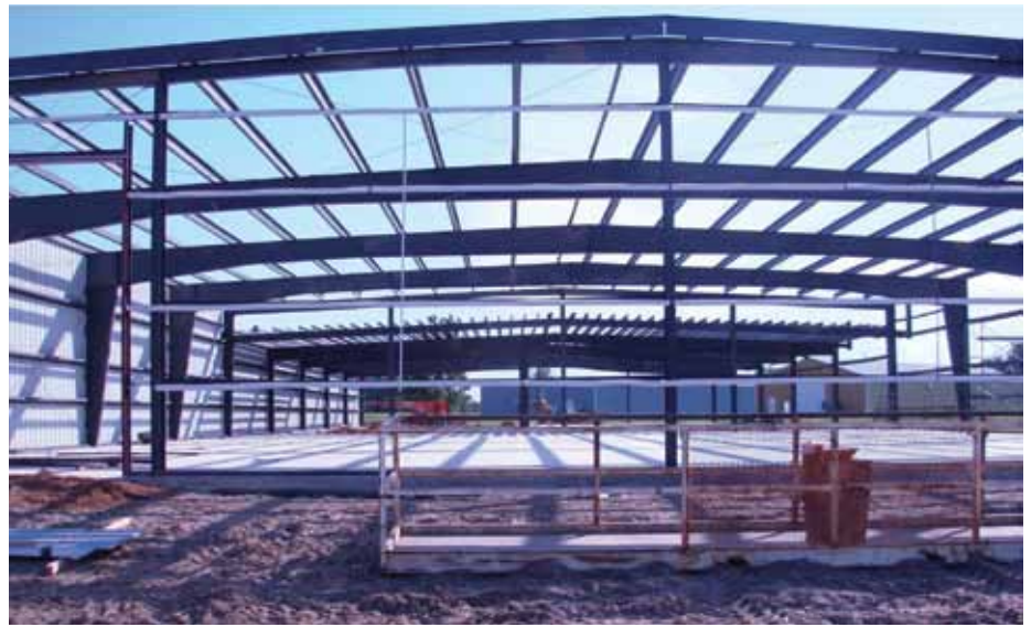
The indoor range was constructed over the spring and summer last year. The large, free-span area will be used to host a wide variety of activities other than indoor archery such as local sport shows, parties and wedding receptions.
